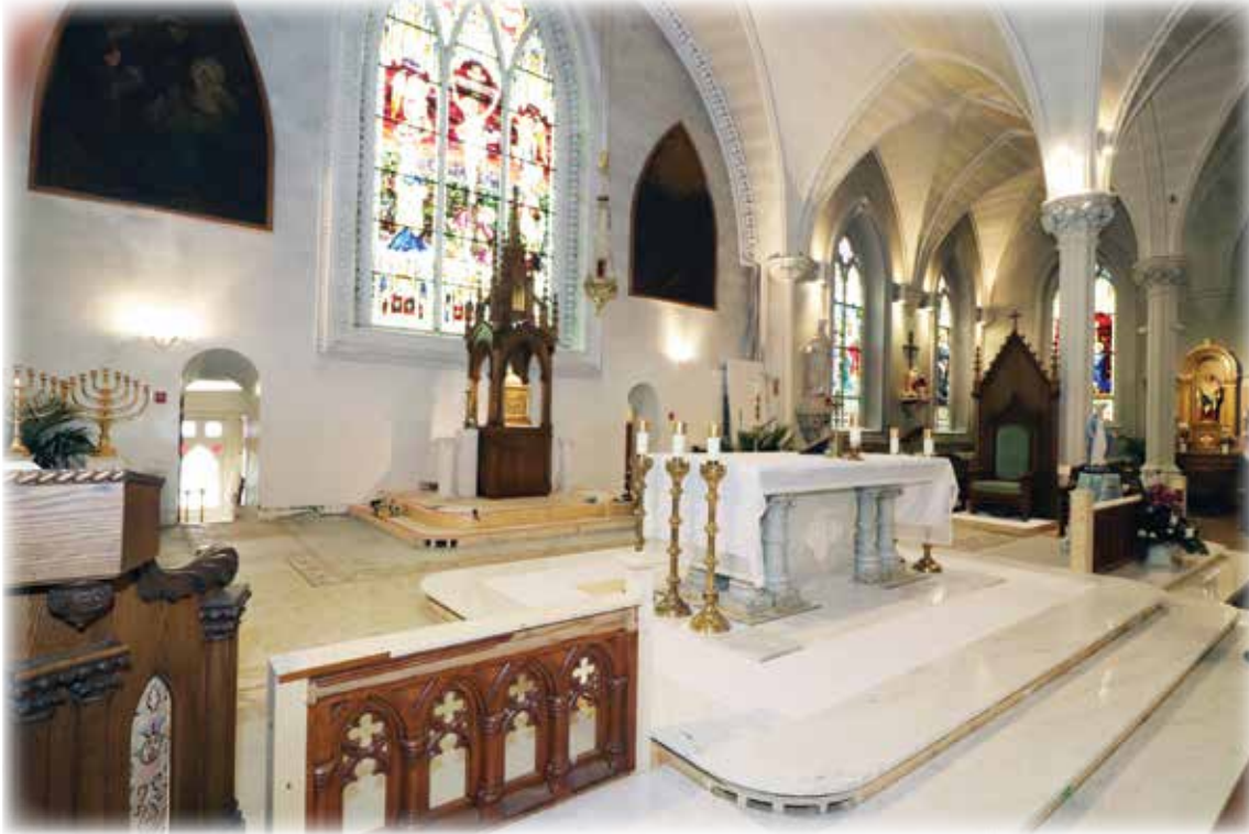
Here we see the work being done on the sanctuary from the west side of the Cathedral.
